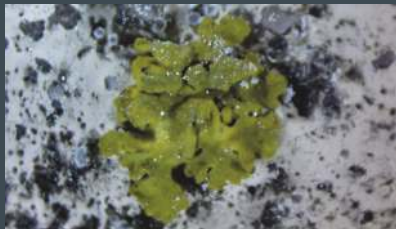
Microbial growth on the exterior of the building
